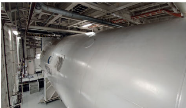
TWIN 295M3 TYPE C LNG TANKS ARE LOCATED AFT OF THE ACCOMMODATION. SOURCE: PHILIPPE HOLTHOF
