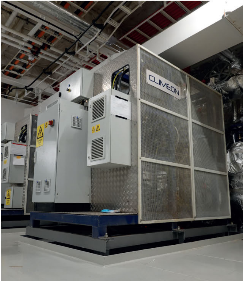
ONE OF CLIMEON'S HEAT RECOVERY UNITS. SOURCE: PHILIPPE HOLTJOF
